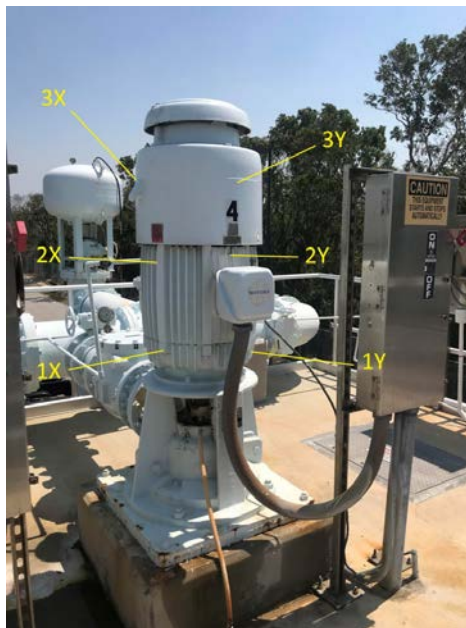
Injection well pump and test points
