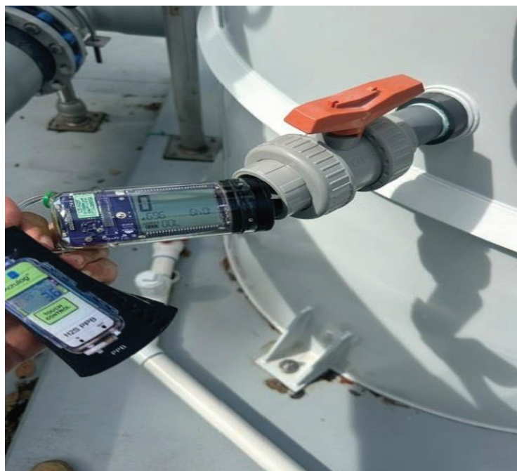
Lower port on in - sink chamber showing 0 ppm
