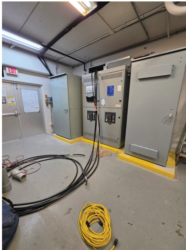
Figure 7: Conductors being routed to new ATS in preparation for the ATS Swap
