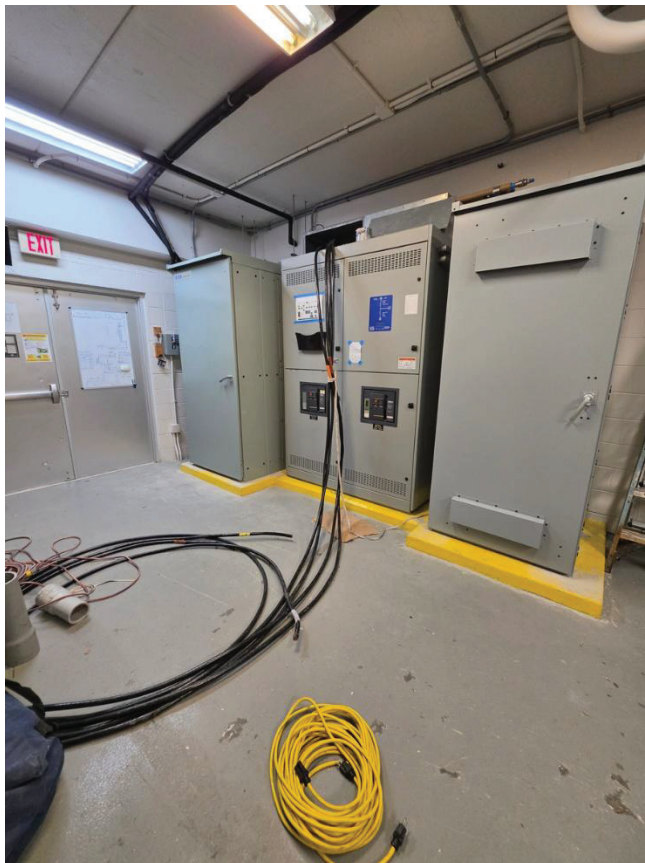
Figure 7: Conductors being routed to new ATS in preparation for the ATS Swap
