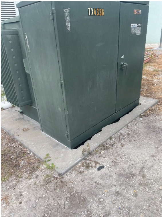
Figure 7: Damaged pad and settling transformer
