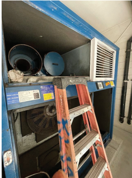
Figure 7: Open blower housing with air filters removed
