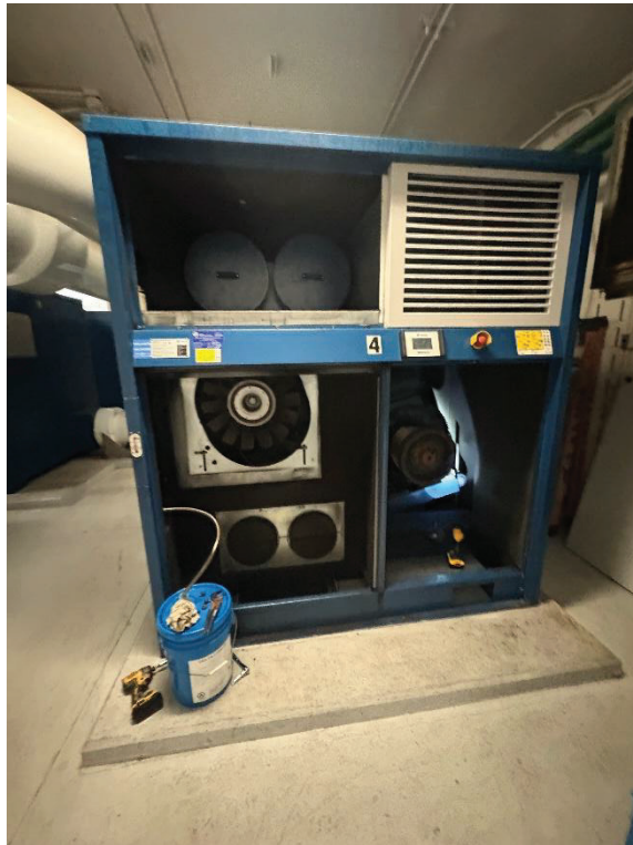
Figure 9: Blower #4 oil draining
