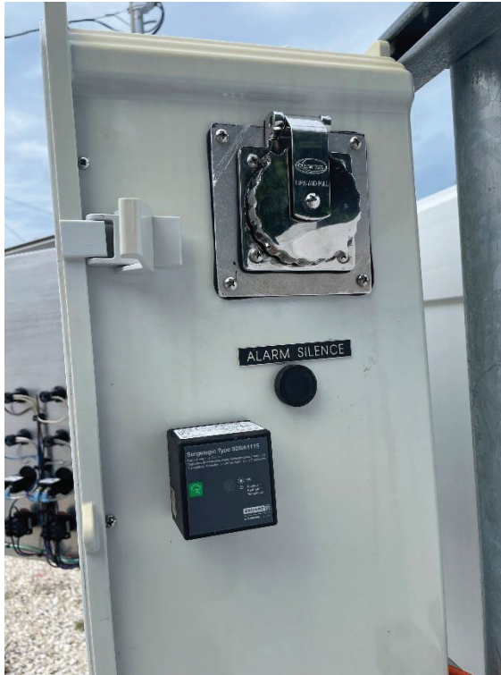
Figure 1: Emergency generator receptacle added to the lift station control panel
