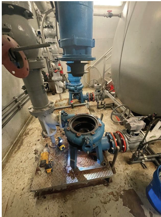
Figure 10: Sewage pump removed from volute and pump base
