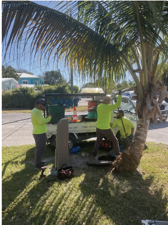
Figure 1. Flovac Crew Installing Vacuum Pit Monitoring Equipment in Basin C (Jewfish Ave)
