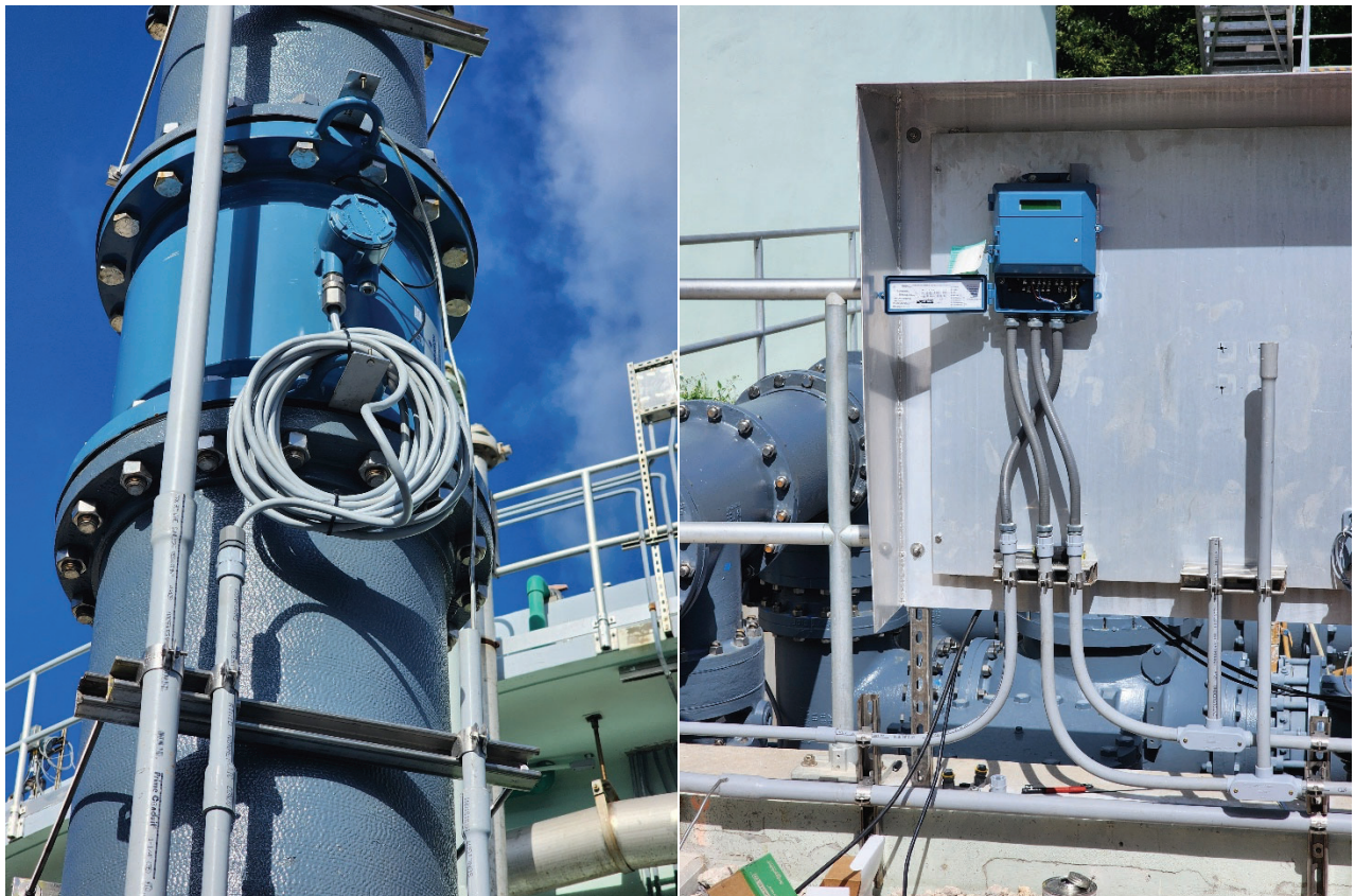
Figure 9 and 10. Conduit Connected to New Flow Meter Display to Flow Meter with Control and Power Wiring
