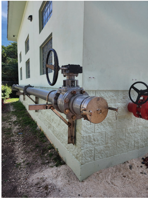
Figure 1. Extended Force main at Vacuum Station A to Front of Building
