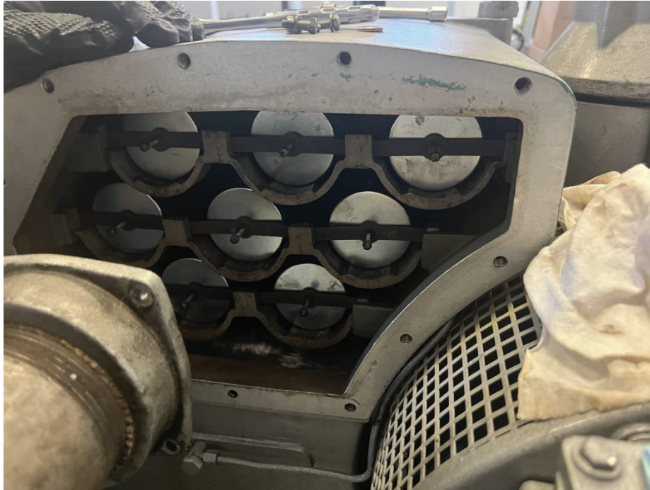
This picture shows the completion of the exhaust filters. Exhaust filters catch the oil vapors and any debris before it turns back into a liquid form and drains back into the return line.
