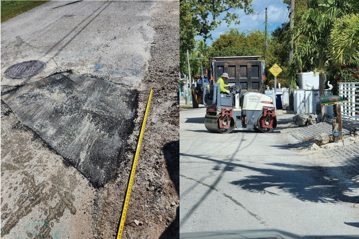
Figure 3 and 4. Compacting Installed Asphalt with Double Steel Wheel Roller/Compactor on #8 Miami Dr.
