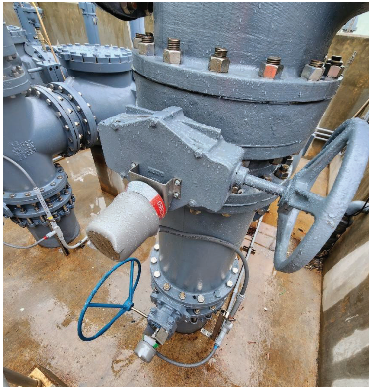
Figure 5. New Valve Position Indicators on Booster Pump Valves
