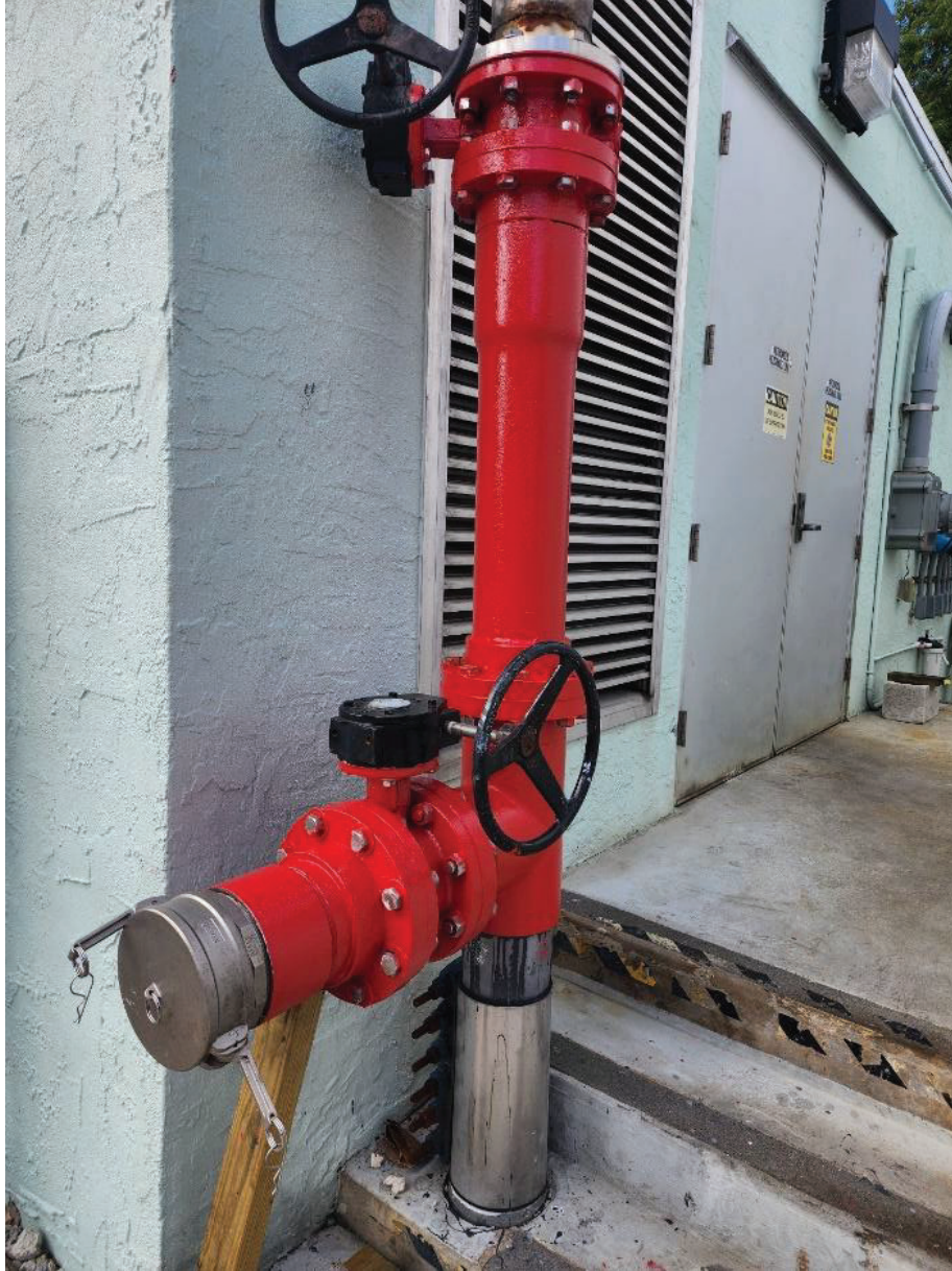
Figure 6. Newly coated odor control piping at Vac E painted in candy apple red from TNE MEC
