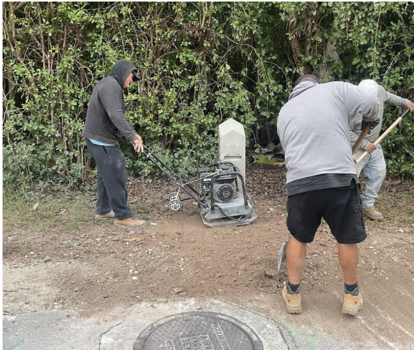
Figure 3. IVC crew compacting the trench with the newly installed conduit, preparing pit for restoration (3/3)
