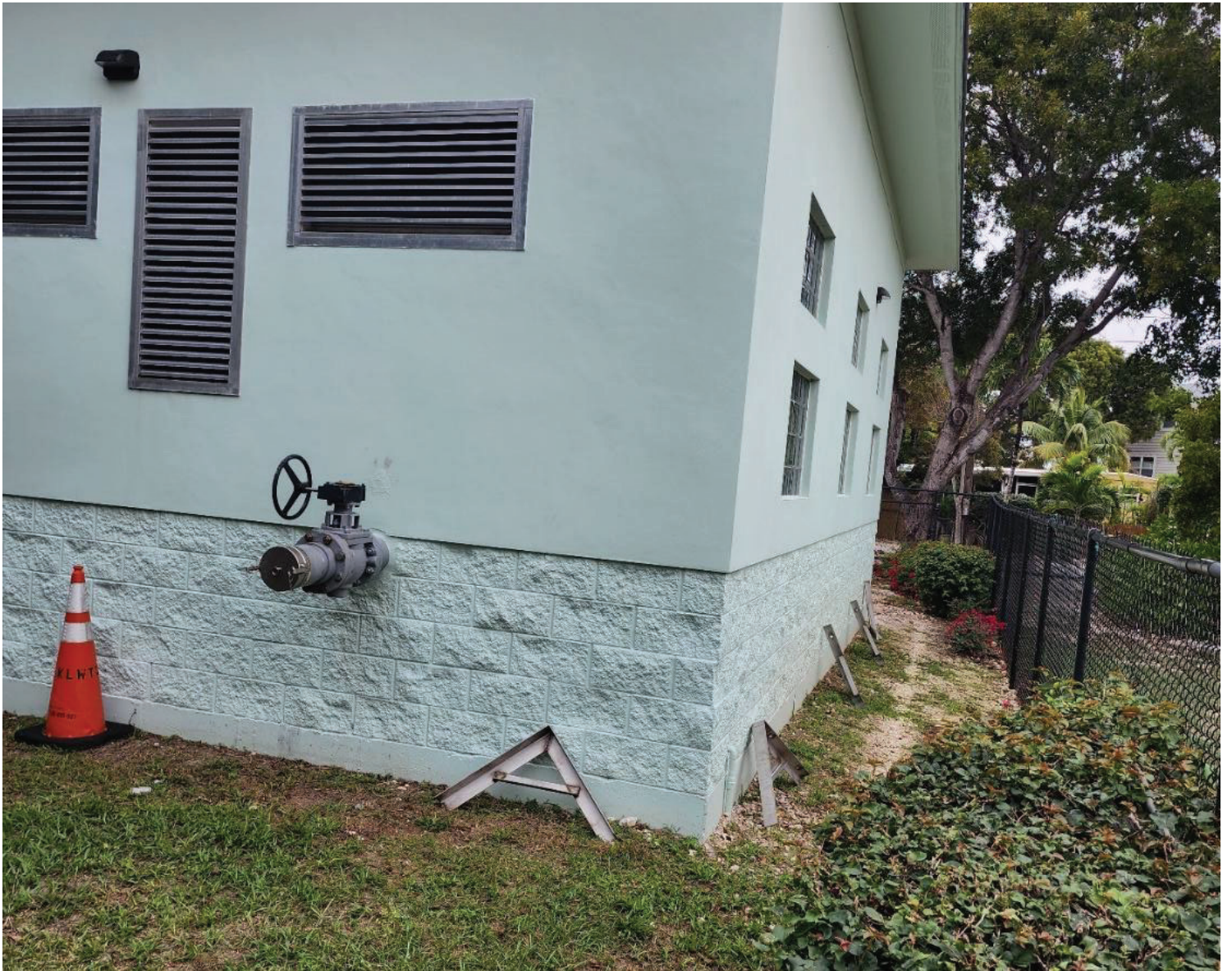
Figure 7. Newly fabricated pipe supports to re-route effluent pipe around to front of building at Vac A
