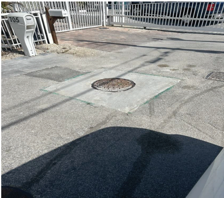
705 Grouper Lane manhole ring damaged and repaired with new ring and 6" concrete slab with rebar reinforcement
