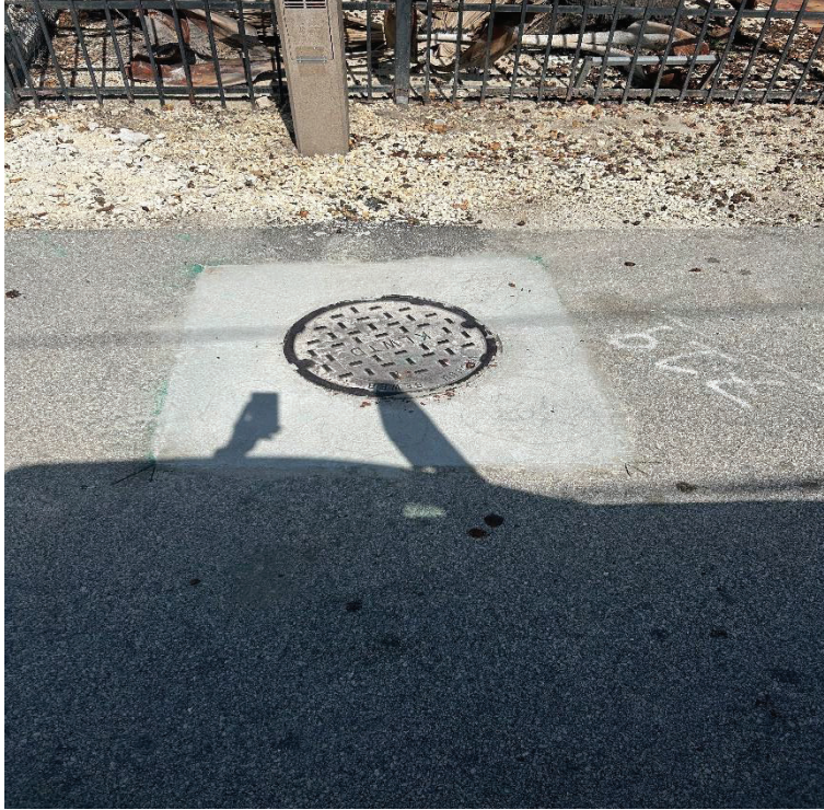
719 Grouper Lane manhole ring damaged and repaired with new ring and 6" concrete slab reinforced with rebar
