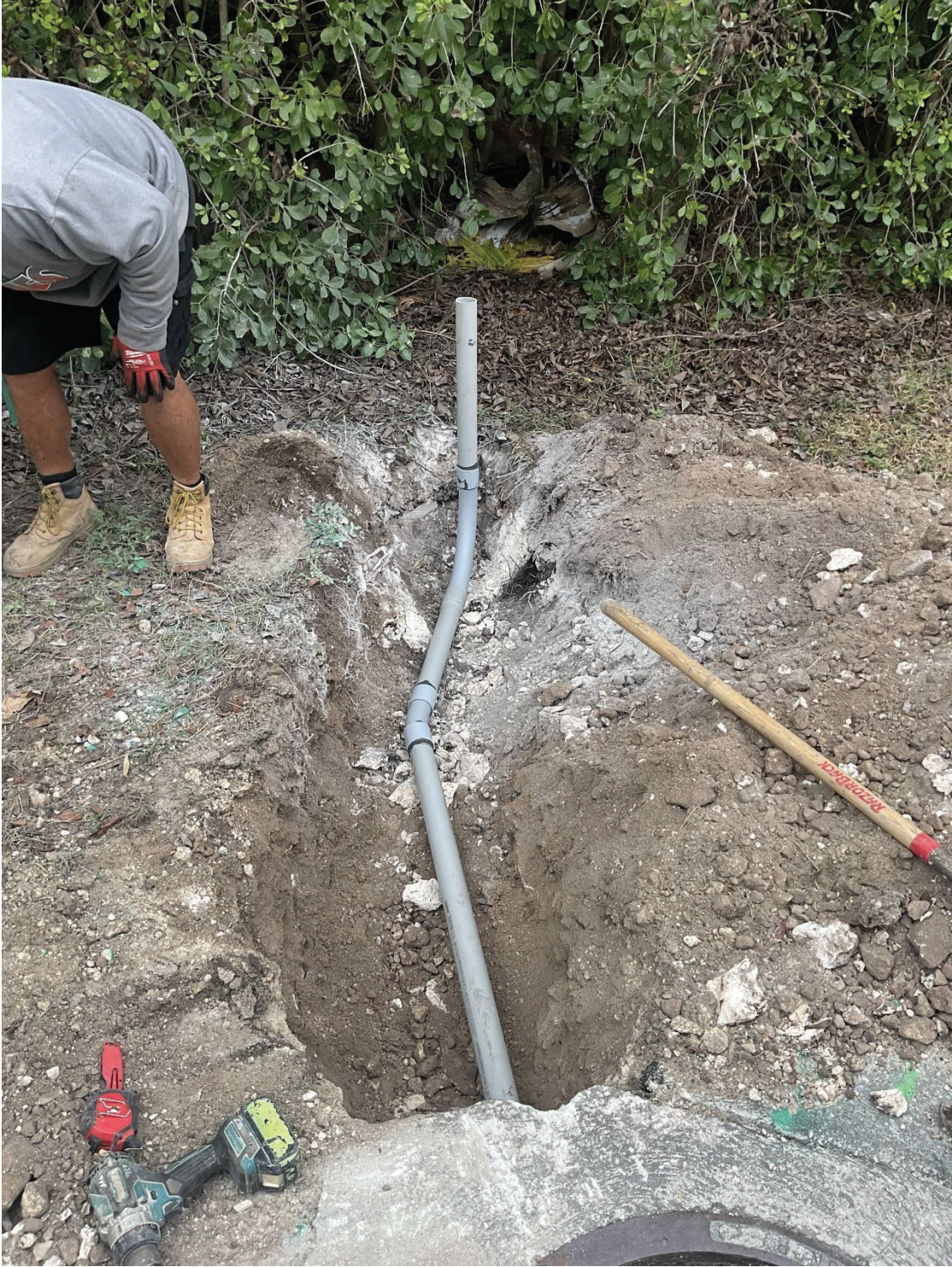
Figure 1. IVC installing conduit in the KLWTD ROW for the Flovac monitoring equipment (1/3)
