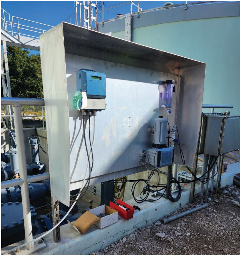
Figure 4. New 316 SS sun shield with turbidity and flow meters installed
