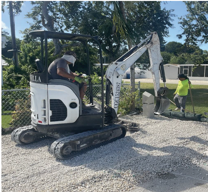
Figure 7 and 8. Installation of Conduit & Flovac Pedestal and Site Restoration for Collection System Monitoring Project
