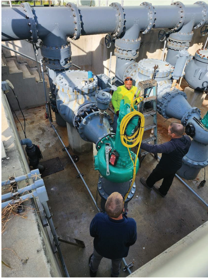
Figure 9. Booster Pump Startup Inspection at WWTP
