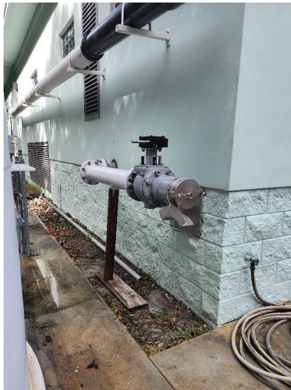
Figure 5. Extended Force Main Connection for Vac Trailer to Corner of Vac G
