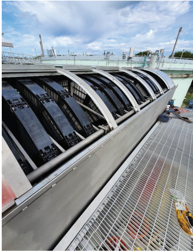
Figure 8. Interior Disk Filters.
