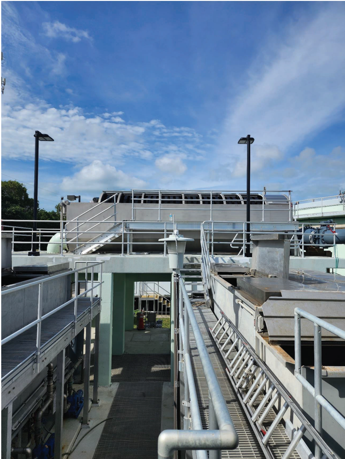
Figure 7. Filter on Platform and Lights Installed.
