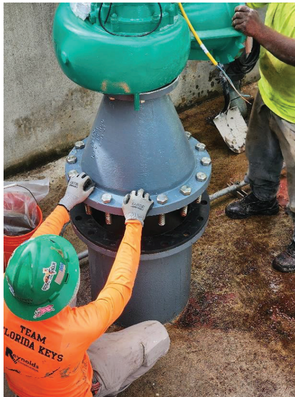
Figure 9. New Booster Pump #4 Installed.
