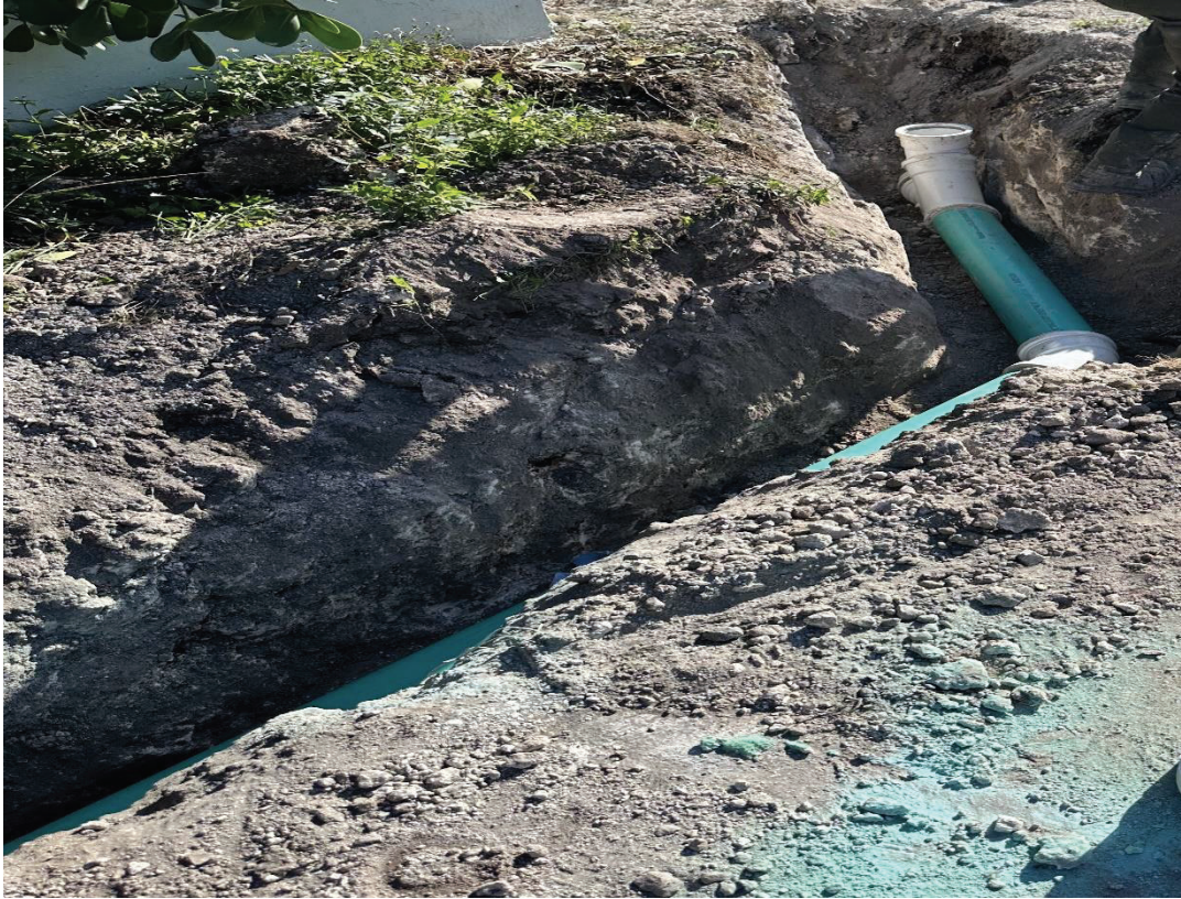
2 Buttonwood Dr add a new clean out service for a new build home.
