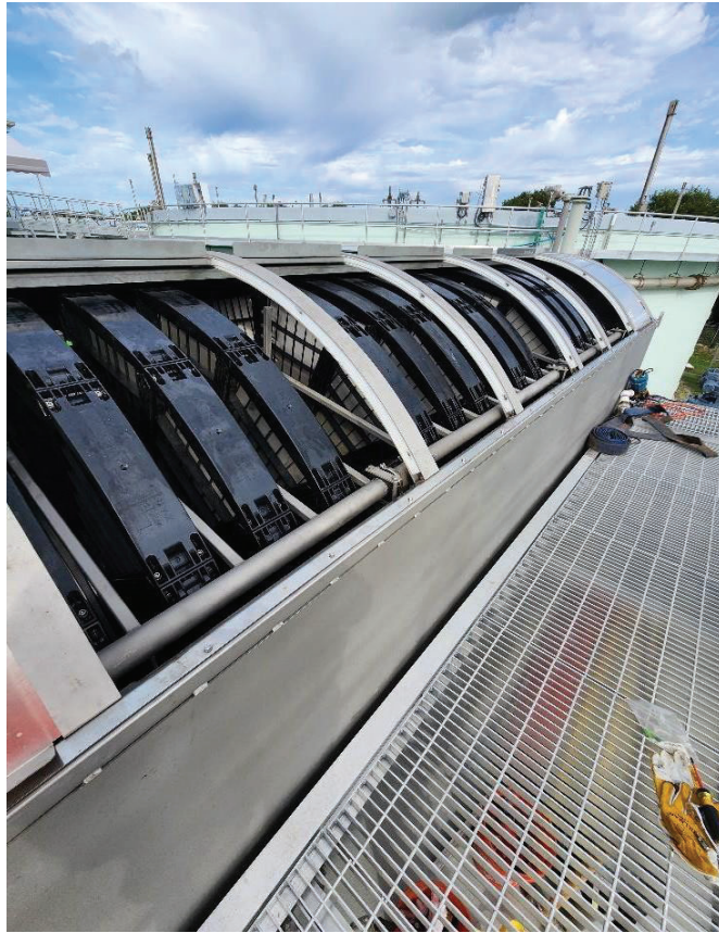
Figure 8. Interior Disk Filters.
