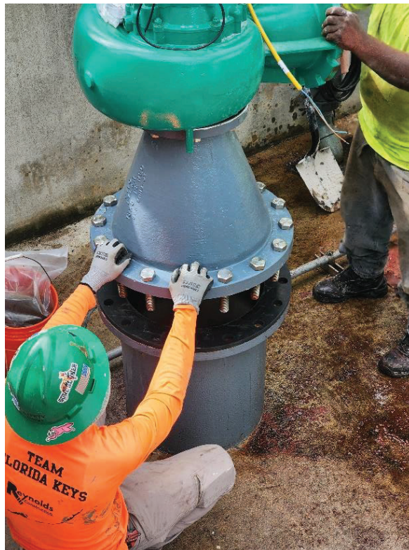
Figure 9. New Booster Pump #4 Installed.
