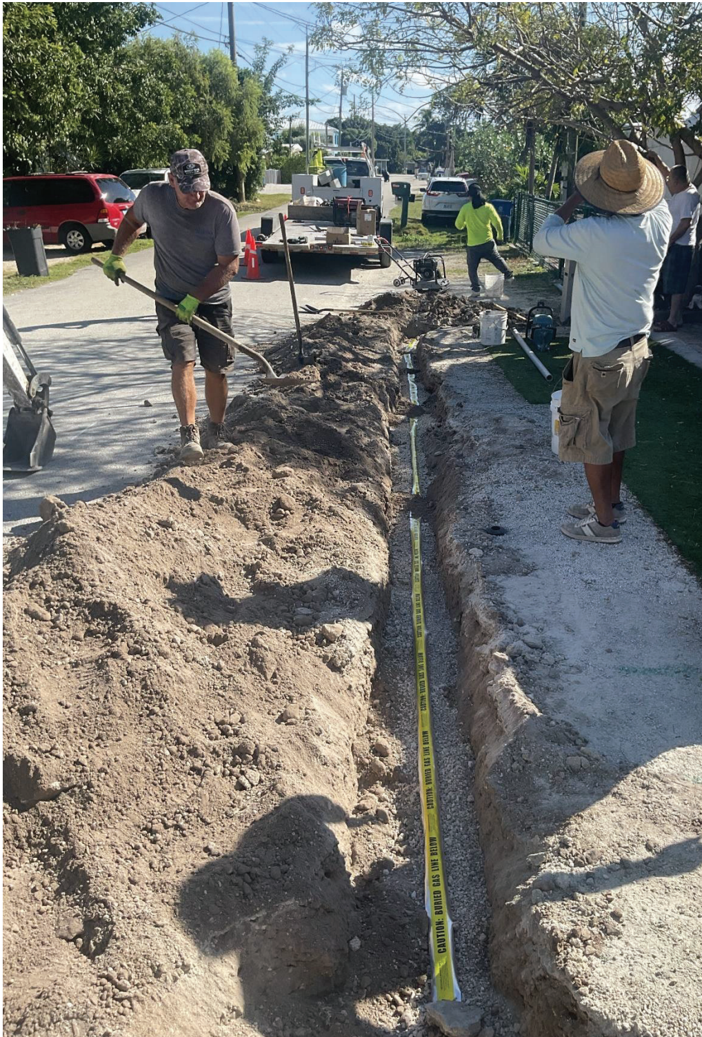
Figure 4. Install Conduit and Detection Tape in Trench for Collection System Monitoring Project.
