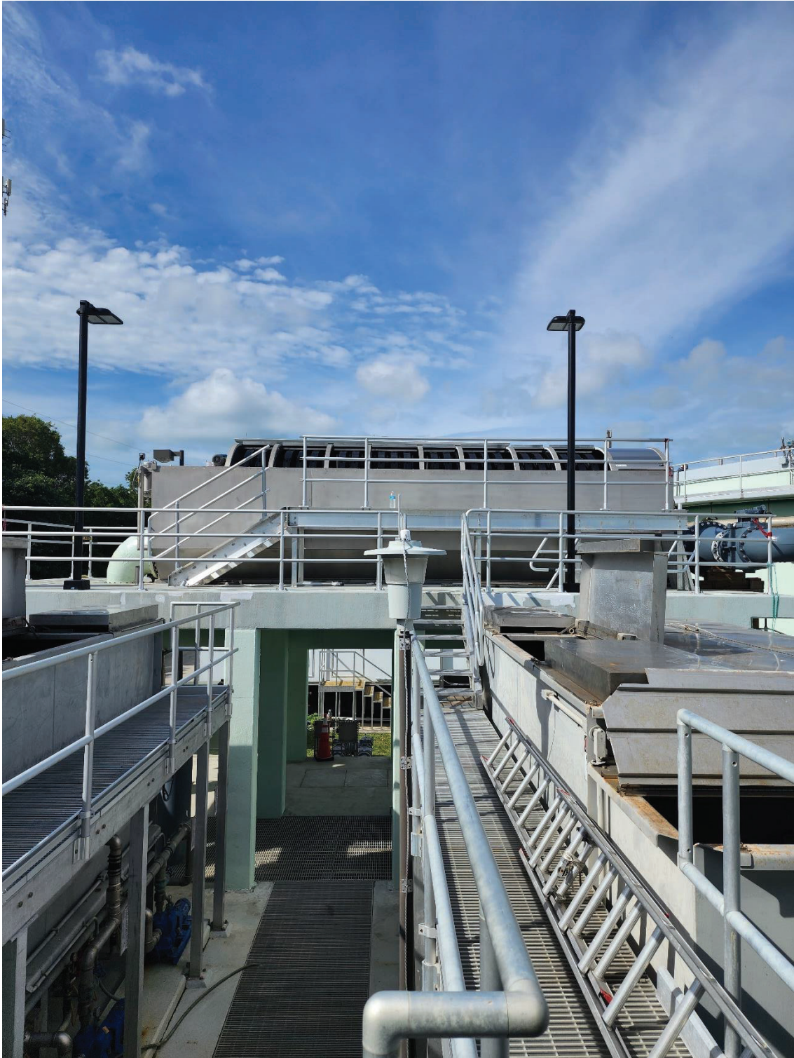
Figure 7. Filter on Platform and Lights Installed.
