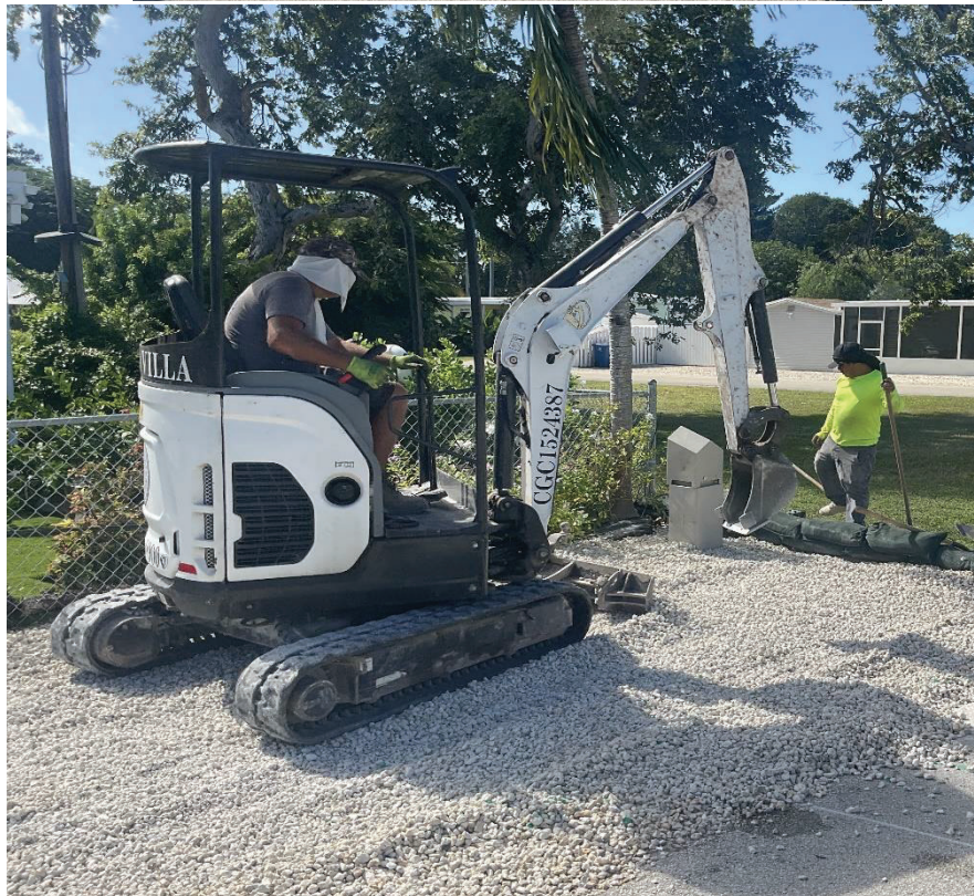
Figure 5 and 6. Installation of Conduit & Flovac Pedestal and Site Restoration for Collection System Monitoring Project.
