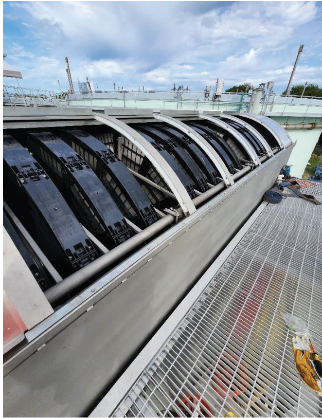
Figure 8. Interior Disk Filters.
