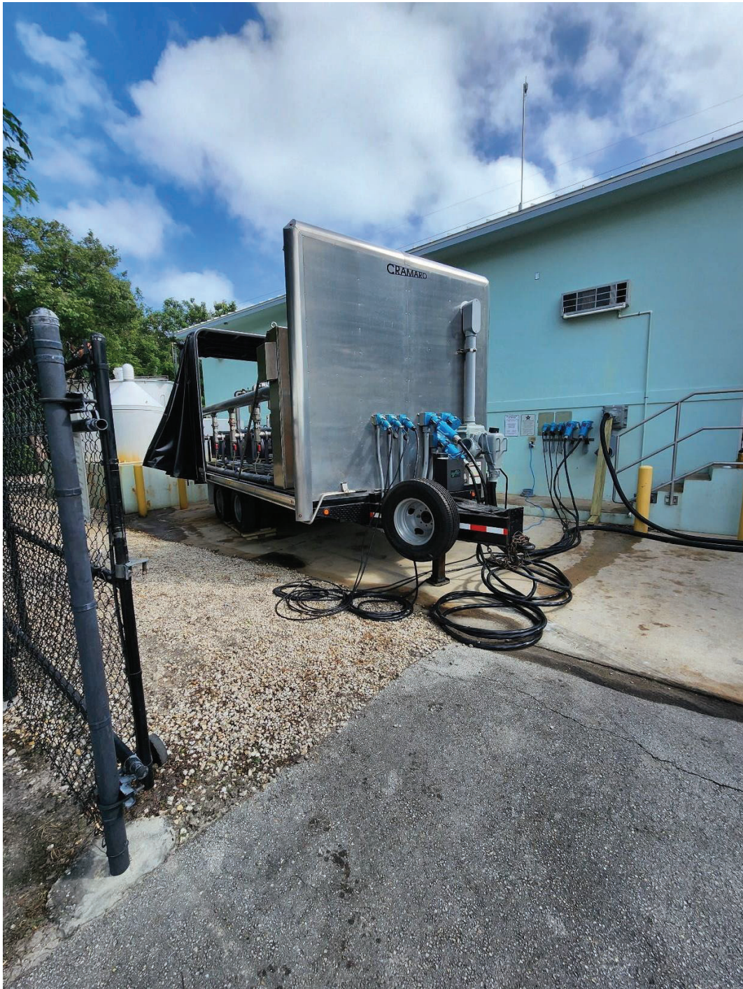
Figure 1. Emergency Vacuum Trailer Connections for VPS Project during Start-Up.
