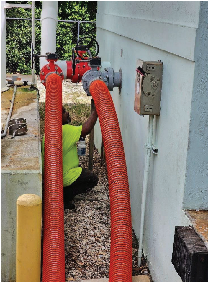
Figure 2 and 3. Emergency Vacuum Trailer Connections for VPS Project During Start-Up.
