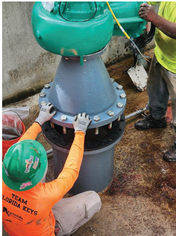
Figure 9. New Booster Pump #4 Installed.
