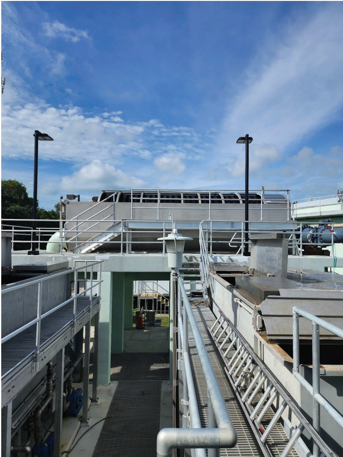
Figure 7. Filter on Platform and Lights Installed.
