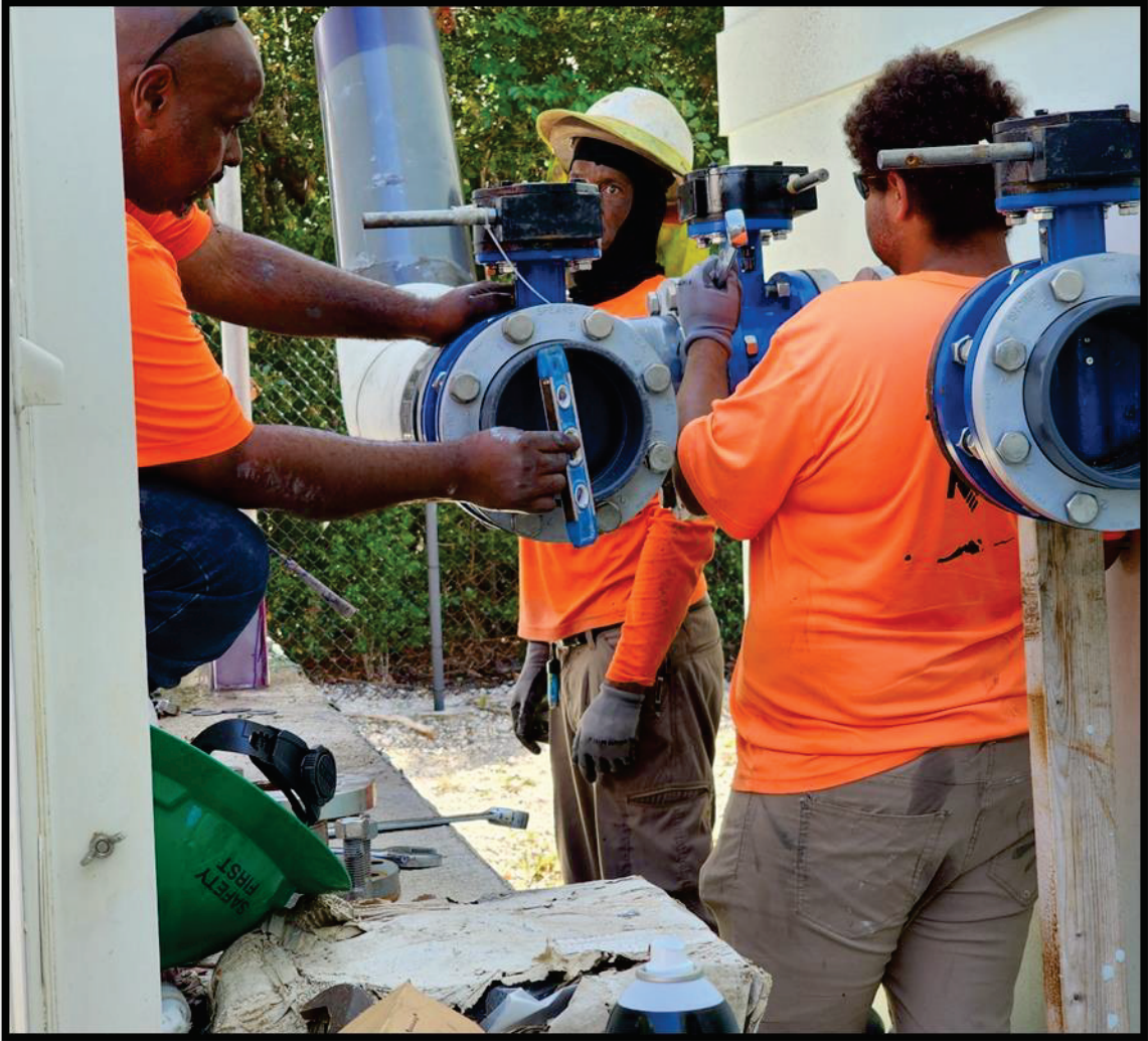
Figure 4: Installing new 8" Butterfly valve, 8"x8" PVC TEE, 8"x6" Reducer, and 6" Plug Valve to Odor Control Piping at Vacuum Station JK
