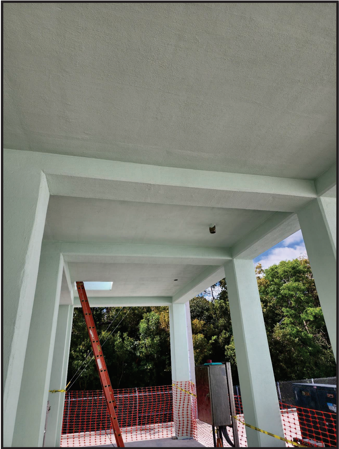
Figure 3: Filter Platform Bottom View
