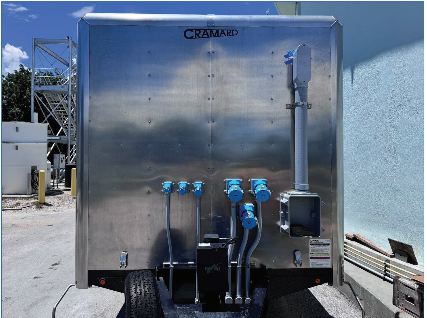
Figure 2: Emergency vacuum trailer front view. Power and control receptacles have been mounted and conduit has been installed.
