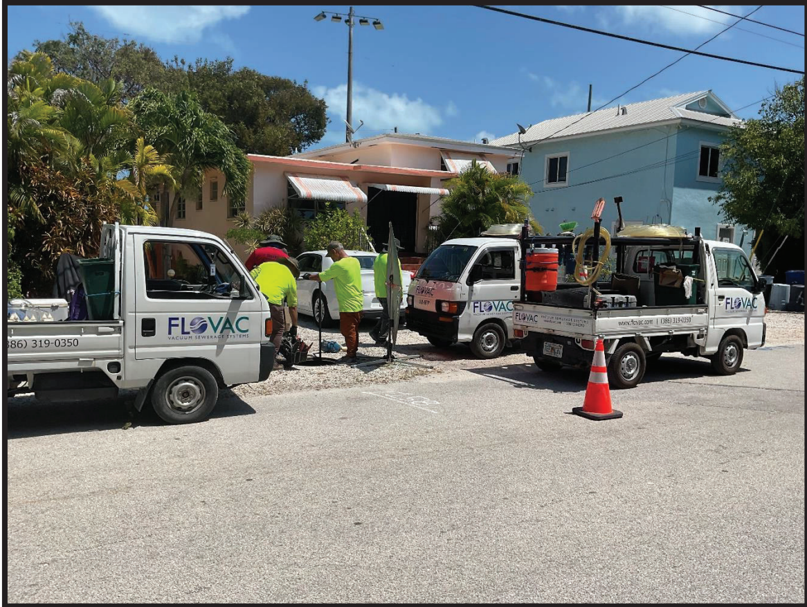
Figure 1: Flovac crew preparing to install monitoring system in a KLWTD vacuum pit
