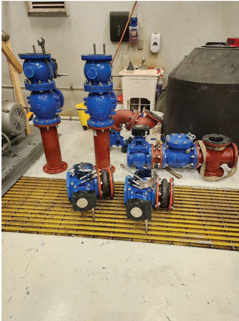
Vacuum Stations Modifications Project: Effluent valves and manifolds assembled and prepared for installation as part of the March 21, 2024 shutdown at Vacuum Station D
