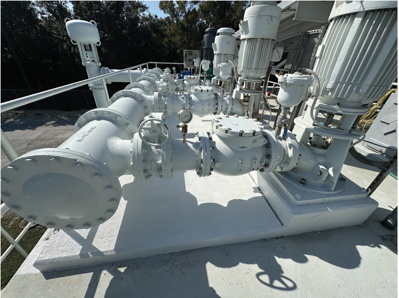
Effluent Filtration Upgrades Project: Coating of the 4" drainage pad at the injection well pumps
