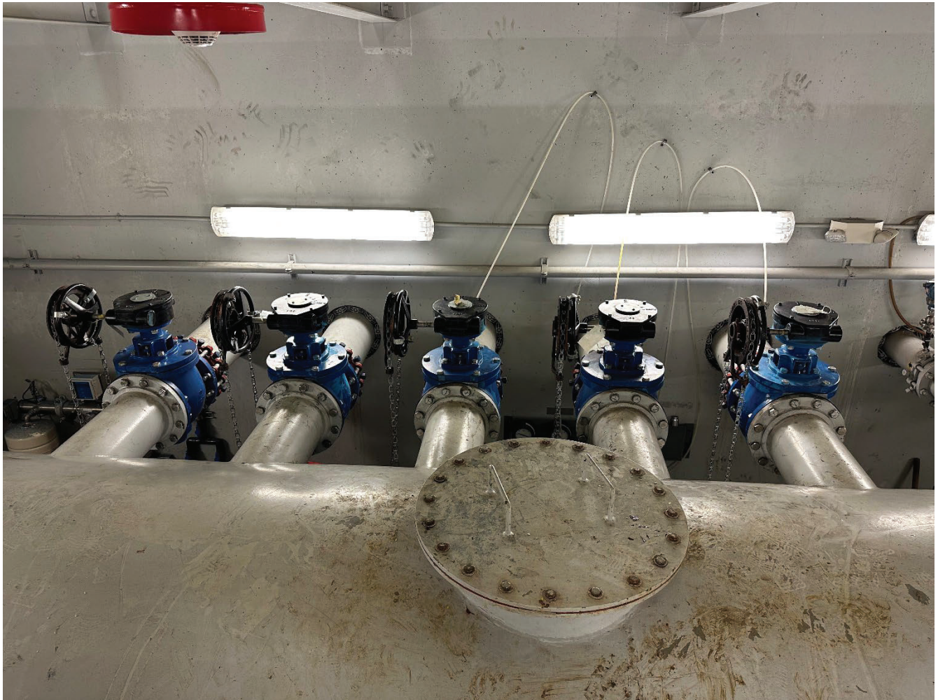
Vacuum Stations Modifications Project: Five new influent ball valves installed during the February 22 nd shutdown at Vacuum Station G.
