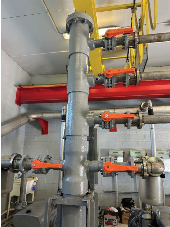
Vacuum Stations Modifications: New vacuum pump pipe tree installed at Vac Station J/K
